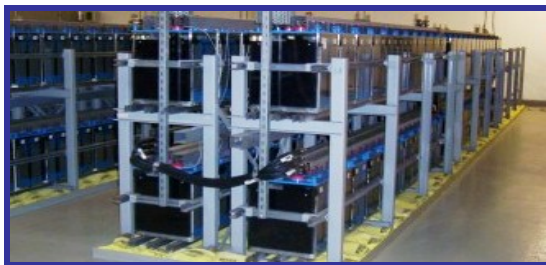
Fig. 2a 20 yr FLA batteries on racks
