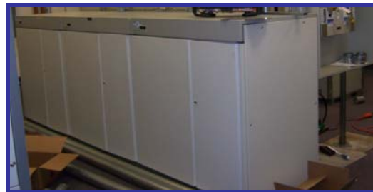
Fig. 2b 10 yr VRLA batteries in cabinets
