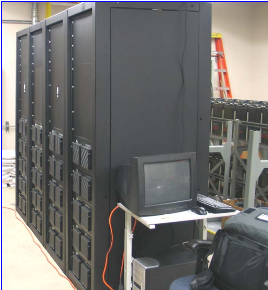
Fig 5. Four rack NiMH system ½ filled. This footprint can accommodate over 1 MW of UPS for 15 second diesel start bridge time applications
