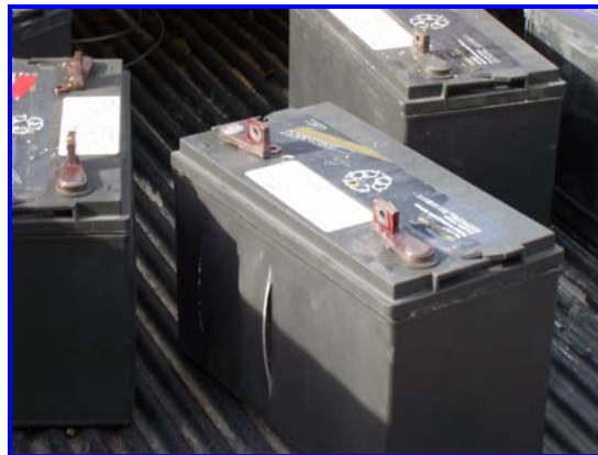
Fig. 2b Failed VRLA battery
