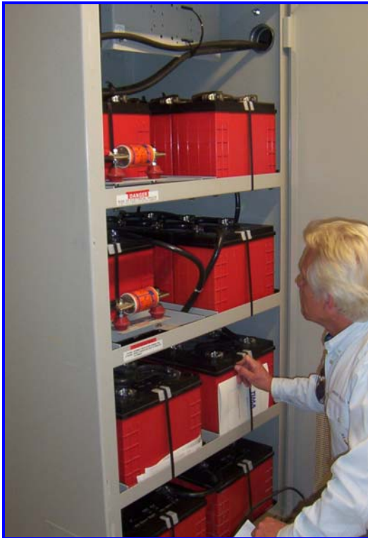
Fig. 2a 3-5 yr VRLA batteries in cabinets
