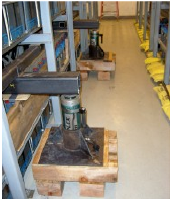
Single rack rams in place
