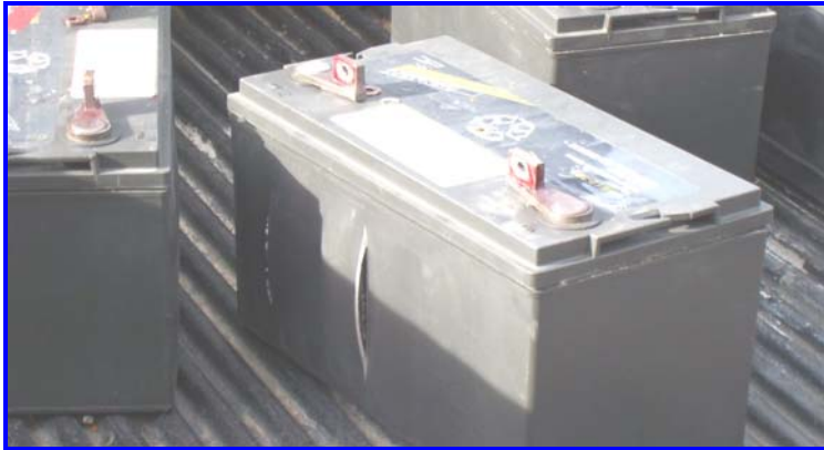
Fig. 2 Failed VRLA battery
