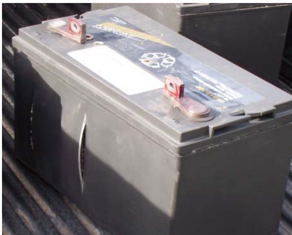
Fig 2 - 6.2 yr old VRLA Monobloc with dramatic failure. Surprising many, no evidence of electrolyte spill here.
