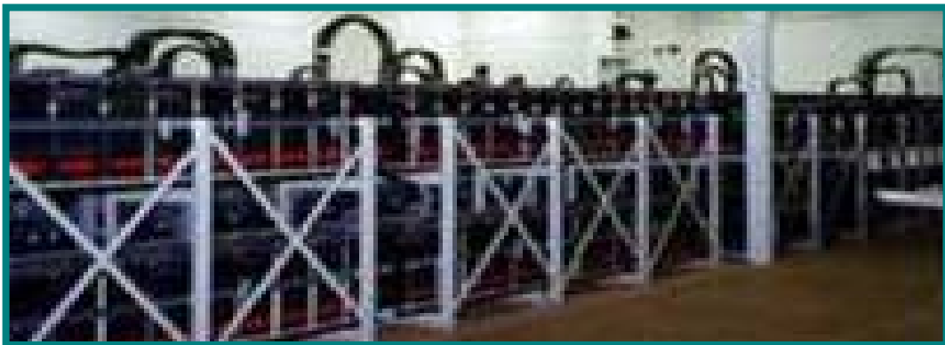
Fig. 1 - Typical flooded cell battery room
